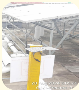
Use of Solar Power for VSS Camera
